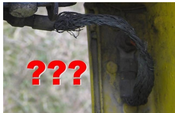
Unacceptable degradation of a bonding strap?
