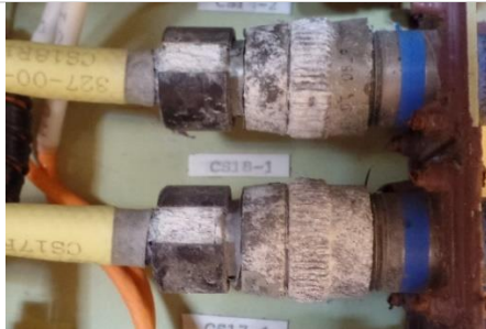
Connector external deterioration
